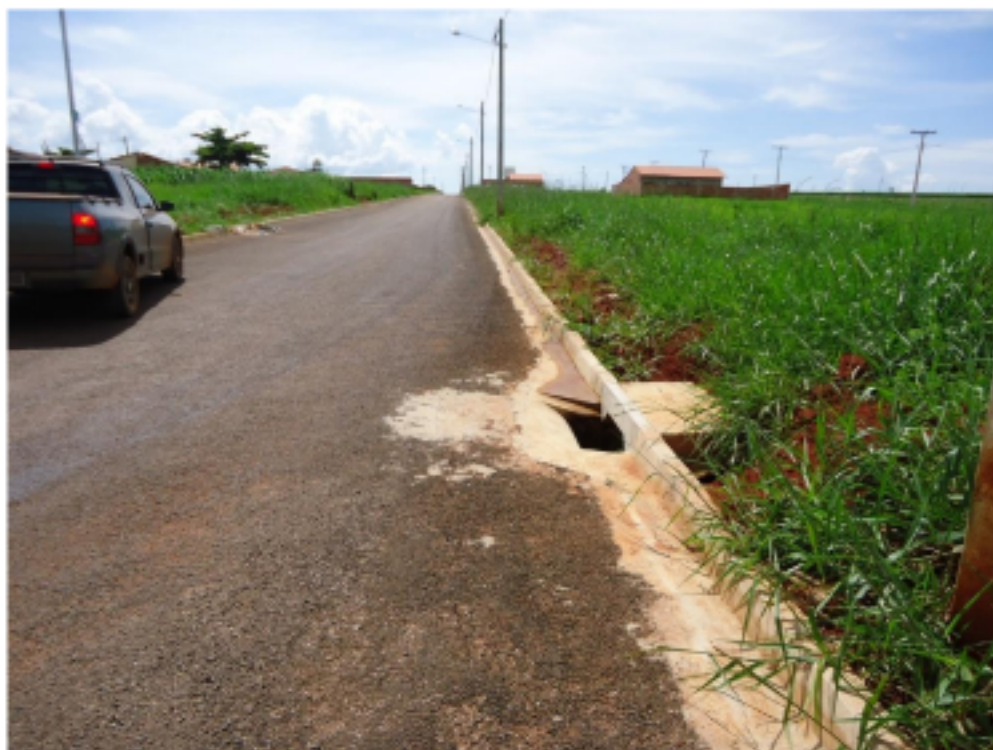
Figura43 - Galeria Pluvial Residencial Dona Zizinha
