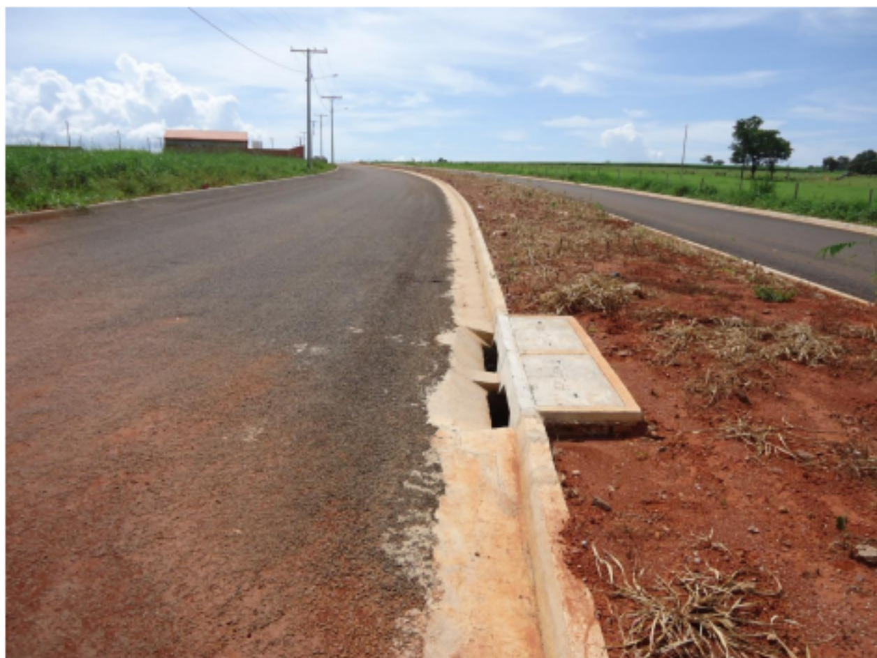
Figura44 - Galeria Pluvial Residencial Dona Zizinha
